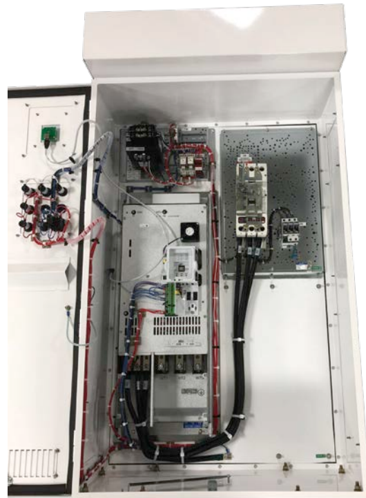
Interior of the PowerXL DG1 three-phase drive pump panel
